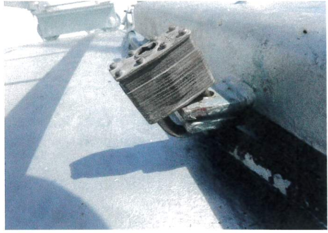
Access Hatch Locked
