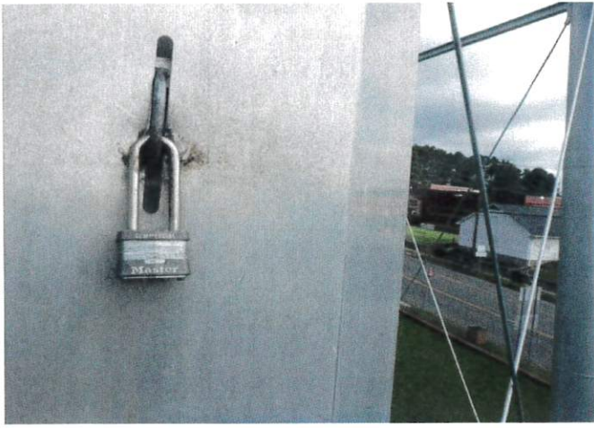
Ladder Guard Locked
