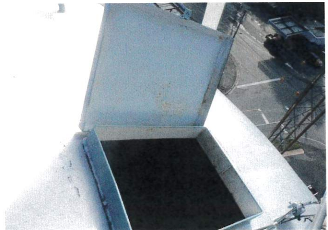
Wet Interior Access Hatch Open
