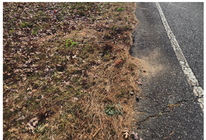
ARV2: Located in roadside depression. (End of manhole hook denotes location of manhole cover.)
